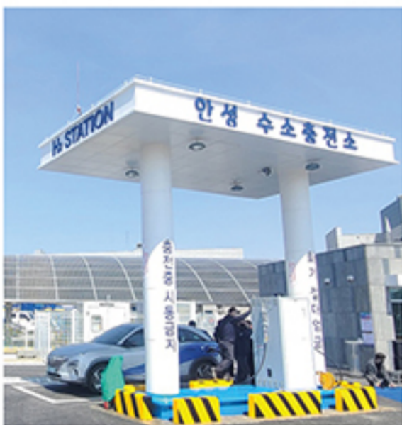
Anseong Charging Station
