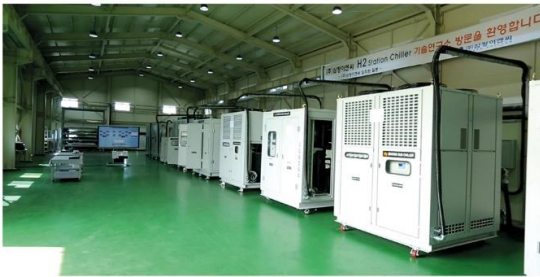
H 2 CHILLER TEST Performance Room
