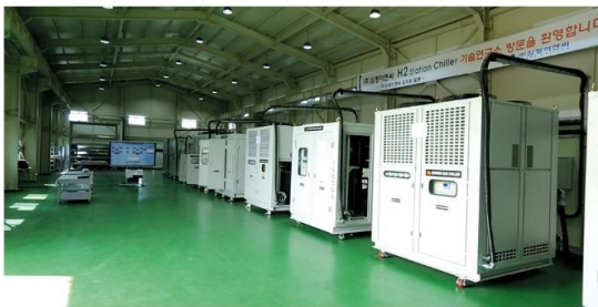
H 2 CHILLER TEST Performance Room
